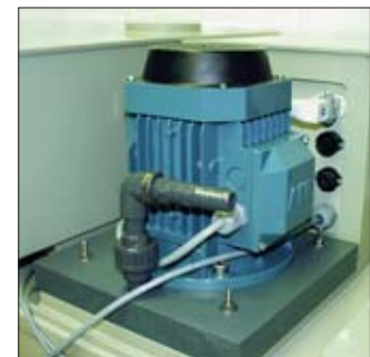
mixer/ pump unit
