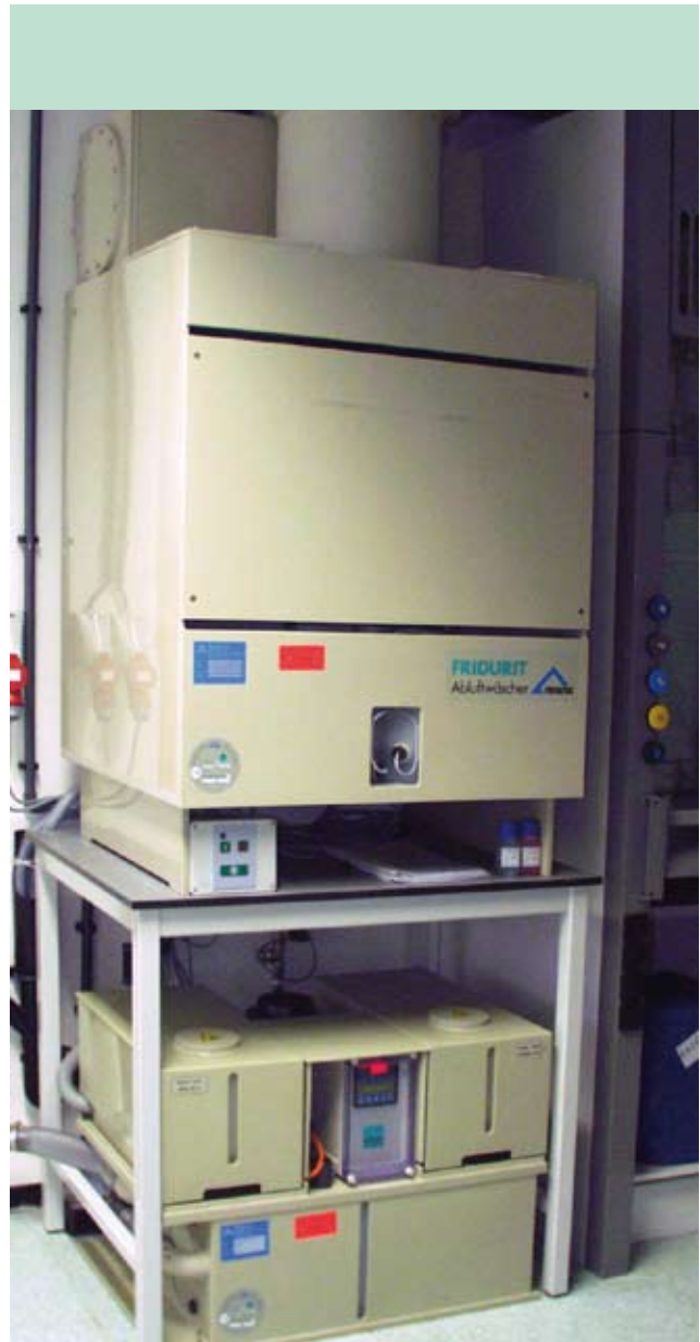
Fig. 10) Fume scrubber C180 and neutraliser unit C100
