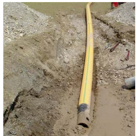
■ Preparation of the insertion of a pipe section into the horizontal flush drilling
