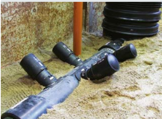
FIG. 15: View into the sewage pipe: Smooth, displacement-free inlets Good inspection capability of the pipes thanks to bright inner layer
